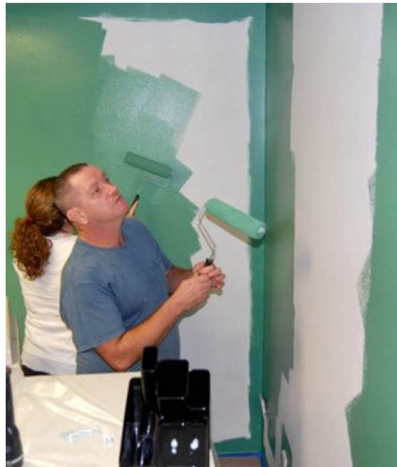
Tim Miller of Somerset adds a coat of paint to an office at the new Isaiah House Drug and Alcohol Recovery Center in Willisburg. (Stephanie Schell photo)
